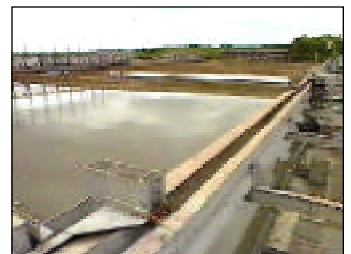
Primary treatment: solids are separated from liquids in a settling tank.
